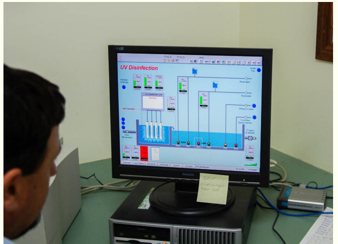
Controls for UV disinfection
